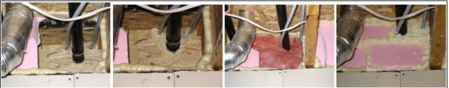
The above photos show a header knocked out to add a laundry tub and the proper re-sealing.
