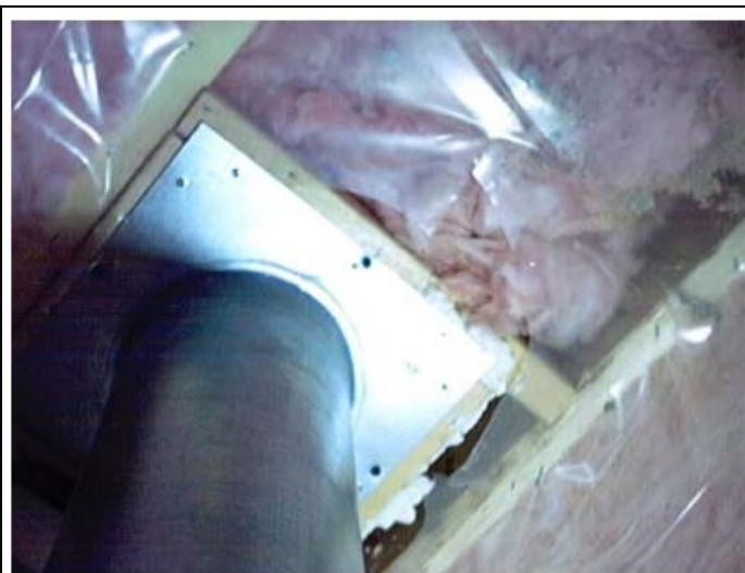
Chimney chases are often leakage areas.
